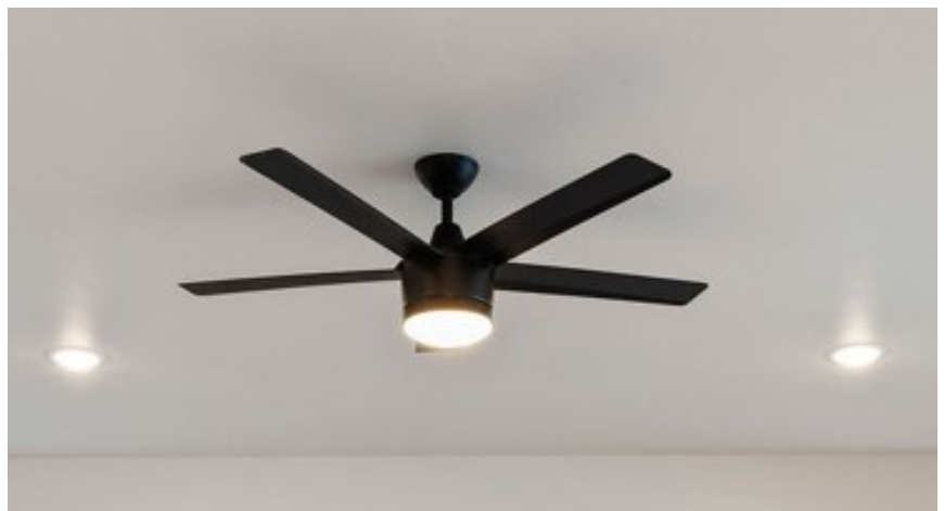
Fan in Great Room and Main Bedroom
